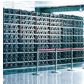
Energy storage system
