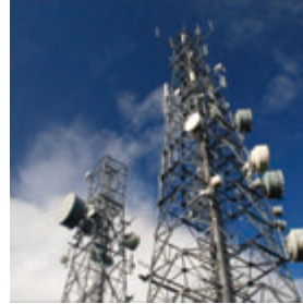
Communication power supply
